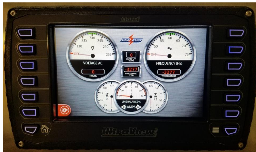
Figure 30 – J1939 Multiplex Monitoring
